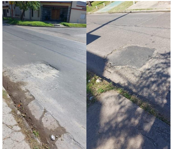
Fig. 10. Pothole at the intersection of Coronel Martinez Street.
