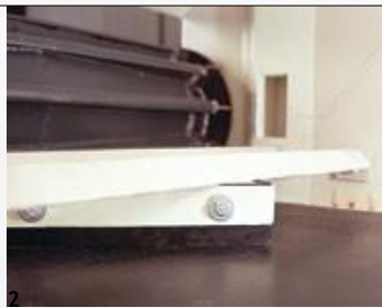
2 V-plow prior to self-cleaning, reloading tail pulley.
