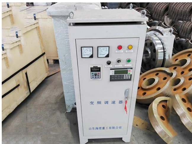
Figura 54, Cabina de control
