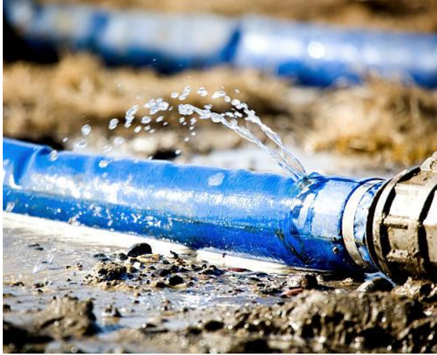
Breaking of pipes in the center of Paraná
