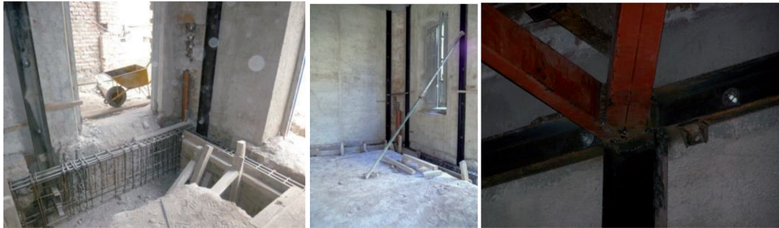
Figure 11. Reinforcement of foundations and reversible metallic structures in columns and lattice, Mitre school, 2012.
