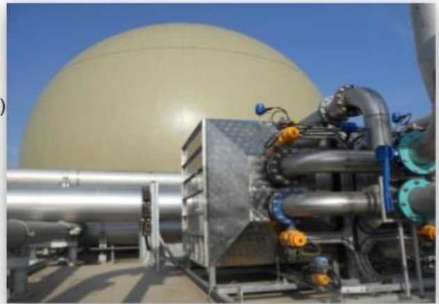
BioGas BGAK on WwTW site.
