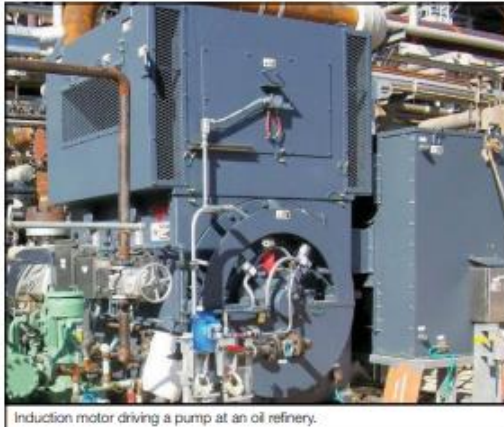
Induction motor driving a pump at an oil refinery.
